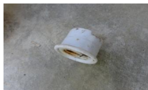
Broken Electric Holder
