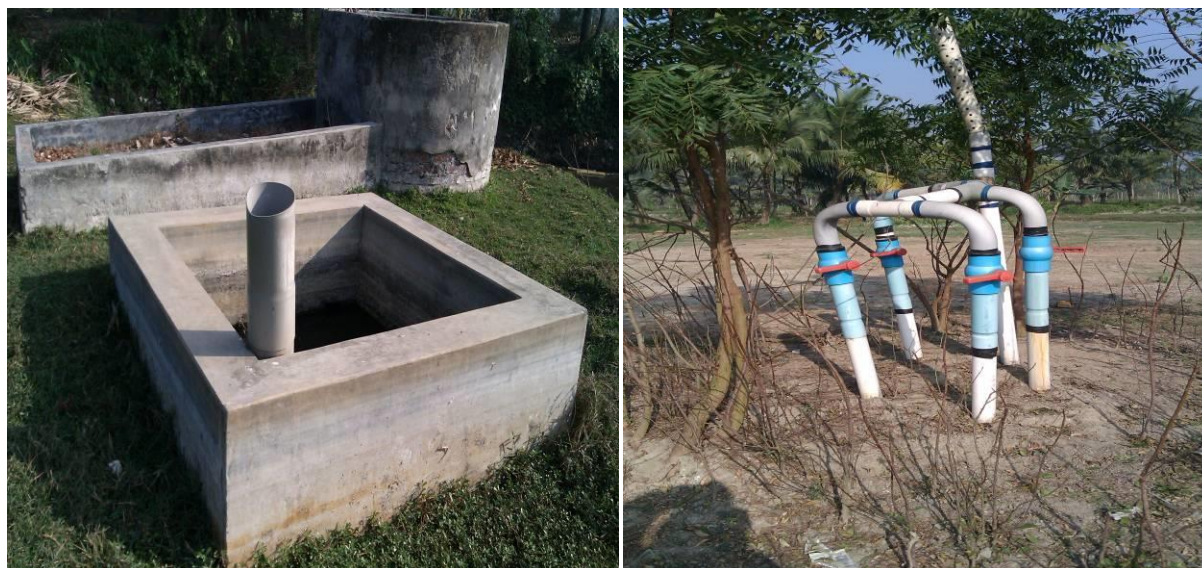
(a) (b) Figure5: (a) leachate collection and treatment tank,(b) Air vent pipe for removal of toxic air
