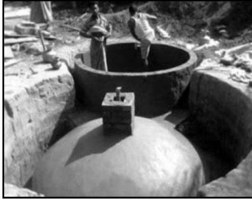
Fig. 6. A Biogas plant
