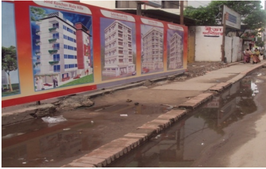
[Fig. 4]. Stagnant water on footpaths
