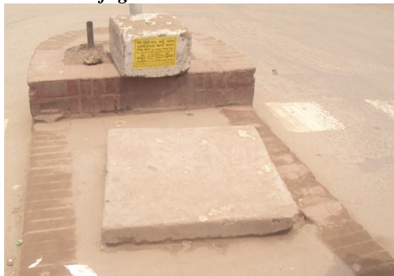
[Fig. 2]. Hazardous pedestrian refuge
