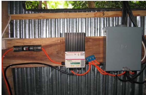
Fig 4. Grid system (Fuse, Charge controller and Distribution box)
