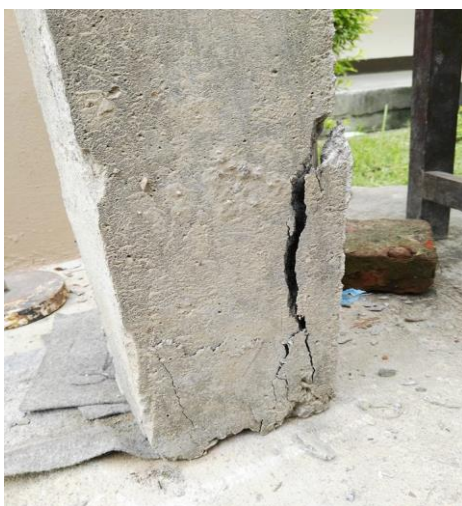
(a) Failure pattern for column containing cement only
