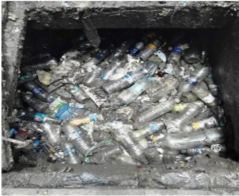
Fig.1 Clogging of drainage system
