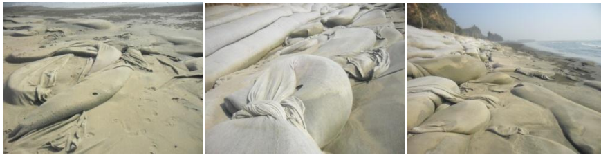
Figure 5: Damaged and burst geotubes.
