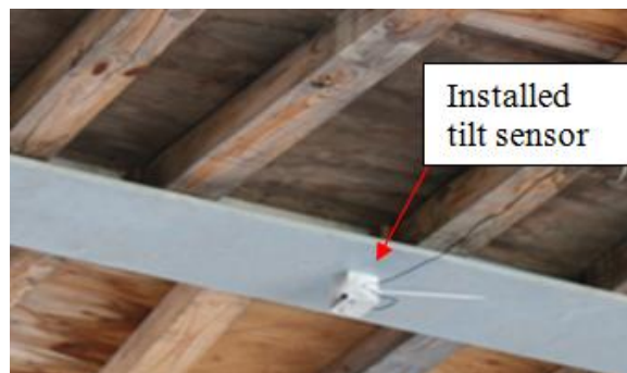
Figure 6: Installed tilt sensor in the bridge
