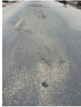
Figure 2: Heave and hump on the surface
