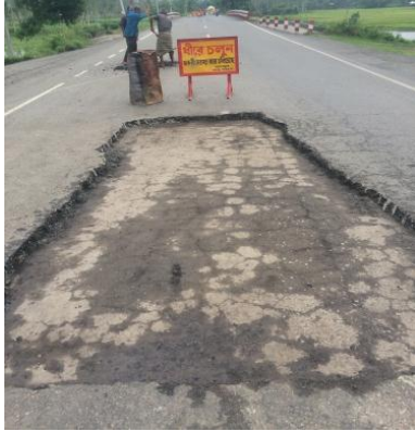
Figure 5: Bottom layer with cracks surface
