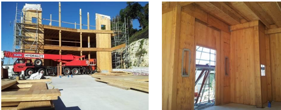
Figure 9: Kaikoura District Council building (left), CLT shear walls (right).
