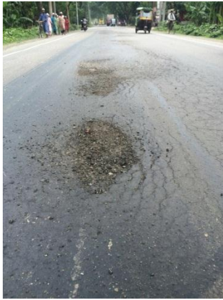
Figure 1: Cracks and Slippage failure
