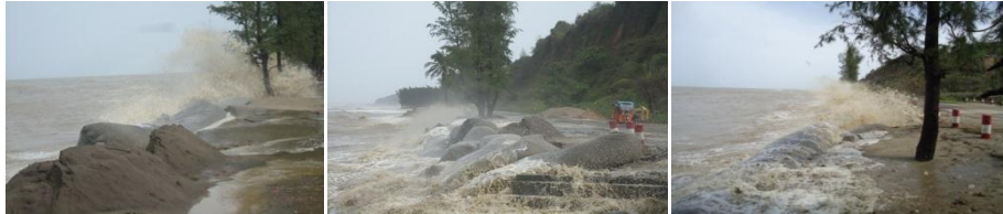
Figure 2: Road affected by tidal surge.
