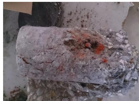
Figure 8: Combine failure occurred
