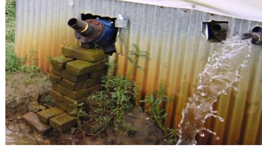
(b) Pumps at operation
