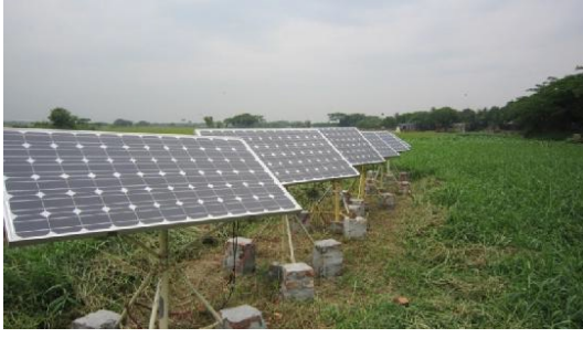
(a) Solar panels at Gaibandha
