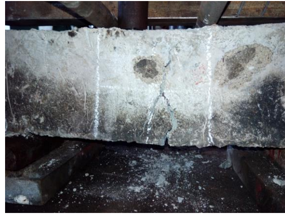
Figure 5: Spalling of concrete in the beam due to burning in fire.
