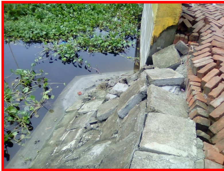
Figure 16: Damages of an approach road of a bridge.
