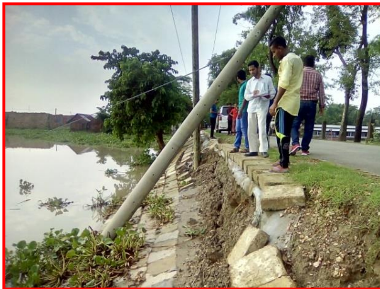
Figure 11. Embankment slope failed.
