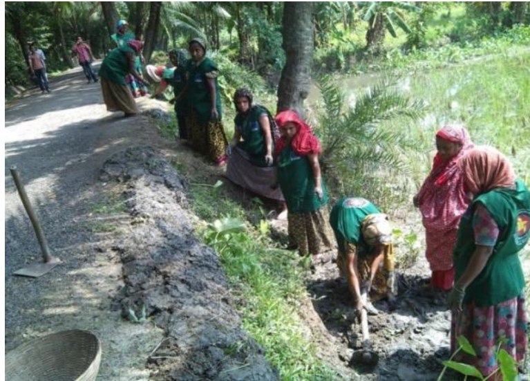
Figure 8: Borrow pit was at the toe of the road. (Location: Babubazar, Barishal).
