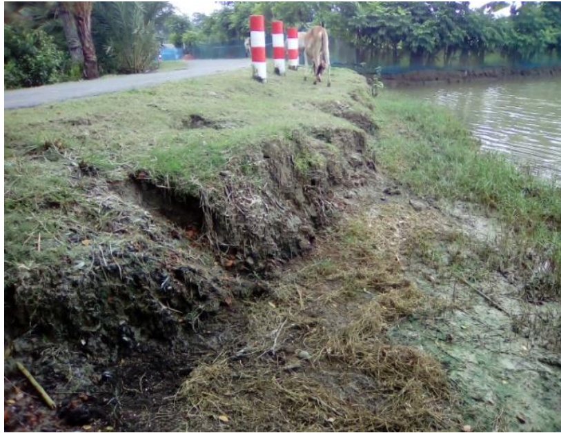
Figure 14: Side slope of rural road washed away by wave action.
