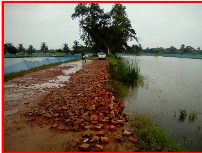
Figure 21: A Portion of road settled
