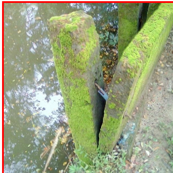
Figure 13: Nut corroded, and Soil washed out in between the plates.
