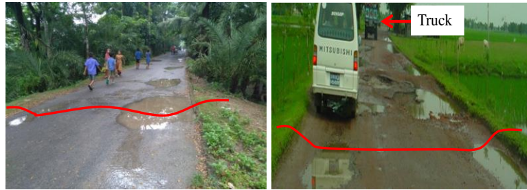
Figure 22: Water logging on the settled pavement and wide spread pot holes
