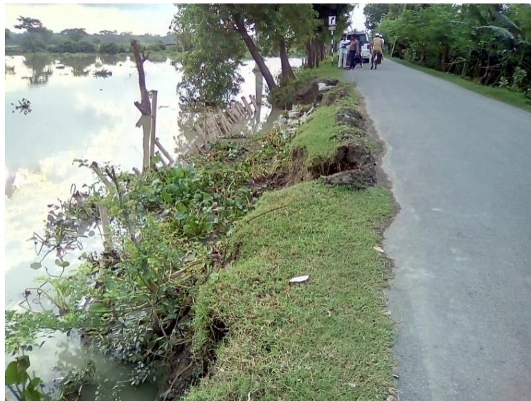
Figure 18: Slope failed in a vegetated slope
