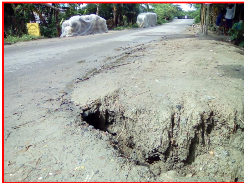
Figure 17: Rain cut erosion in shoulder without vegetation
