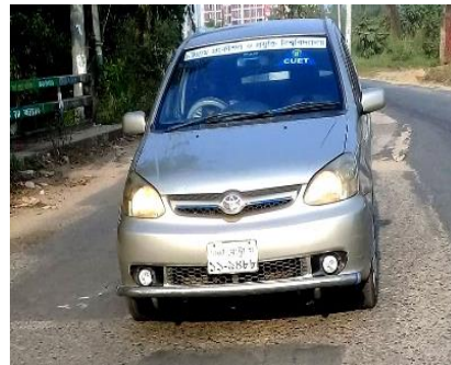
c) Very poor road pavement condition
