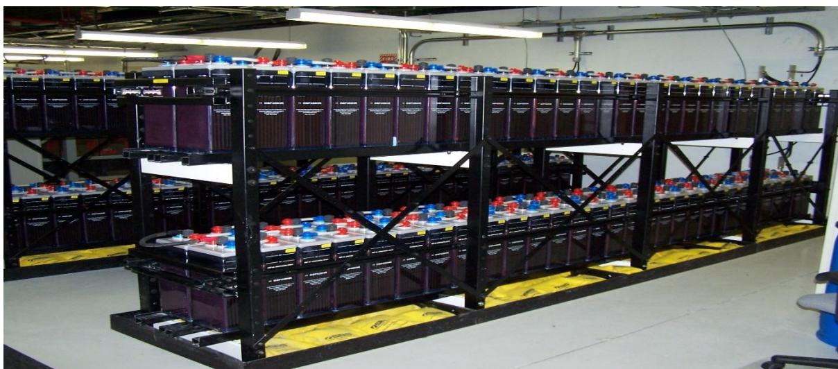
Figure 3.22:- Battery Bank System
