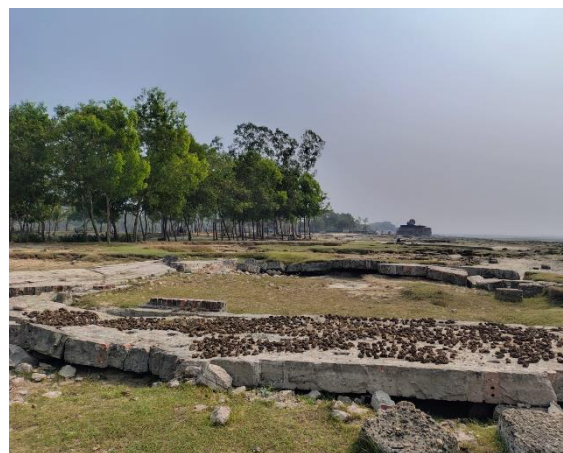
Damage to buildings due to Coastal erosion
