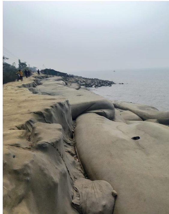
Damage embankment due to coastal erosion
