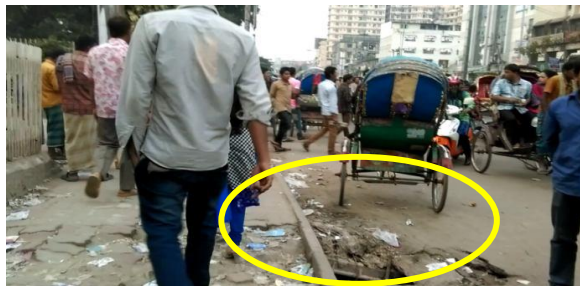
Poor Quality of Walkway (New Market area)
