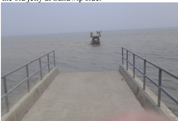
Photo: 1 Damaged BIWTA Jetty at Sandwip side at high tide (September, 2014)
