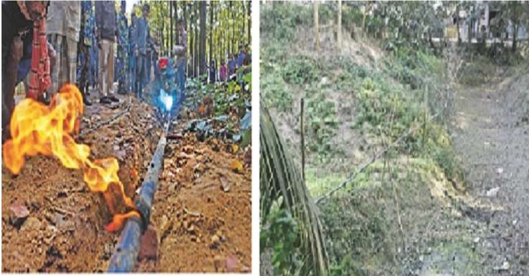
Figure 04: Illigal gas connection never flow the Rules and Regulation. [4, 20]
