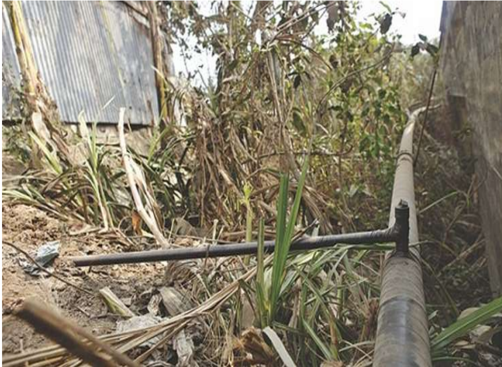
Figure 03: Illegal Gas Connection never flow the Rules and Regulation [4]
