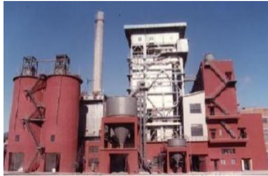
FIGURE 15 130t/h CFB boiler with improved square cyclone.
