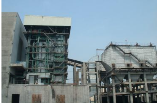
FIGURE 14 75t/h CFB boiler with improved square cyclone
