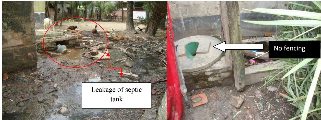
Figure 5: Problems in sanitation facilities in jogipole union.
