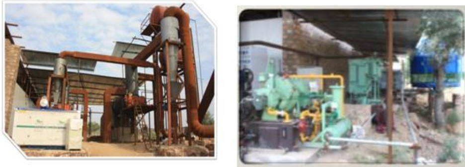
Fig. 4: Biomass Boiler, Turbine and VAM Set Up
