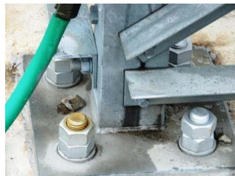
Fig. 2. Base of circuit breaker anchored by bolts
