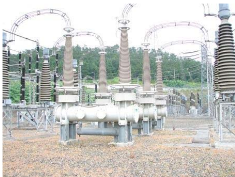
Fig. 1. Circuit breaker in Switchyard
