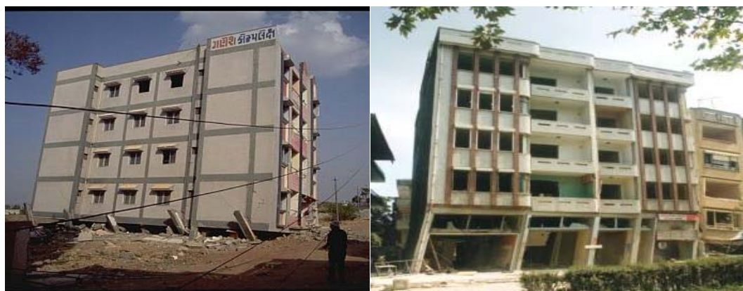
Fig. 2 Failure of structures associated with soft story under earthquake (From Google image)
