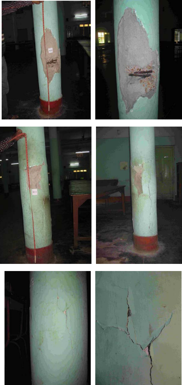
Figure 7: Photograph of some damaged dining hall columns
