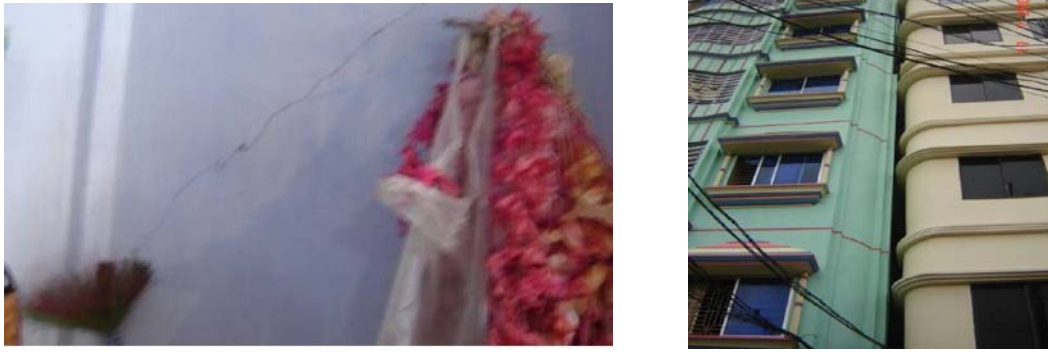
Figure 1: Photograph of some affected buildings in Rajshahi district after the earthquake on July 5, 2008
