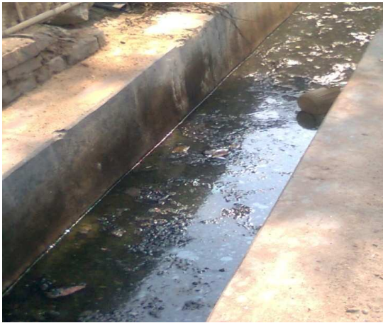
(a) Flow reduced due to garbage at Munsi Para
