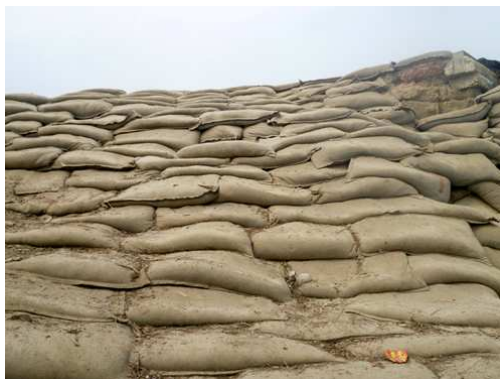
(a) Geobag revetment
