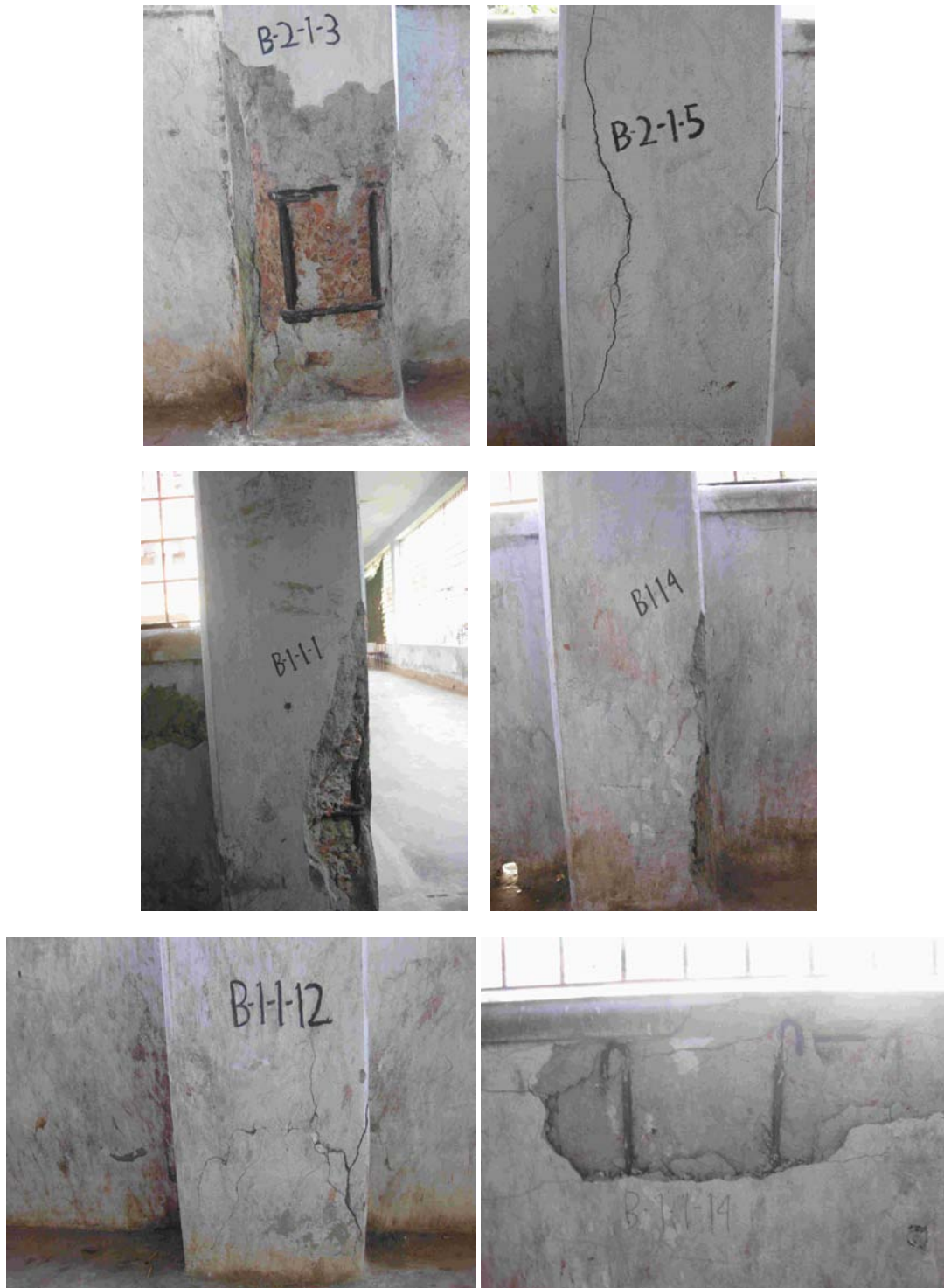
Figure 8: Photograph of some damaged parts verandah column and part of railing
