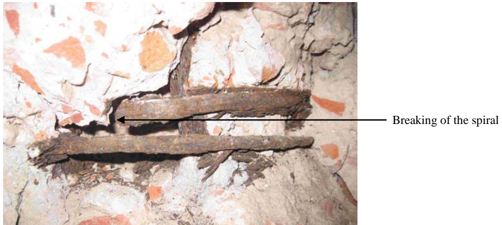
Figure 9: Breaking of the spiral bars of dining hall column
