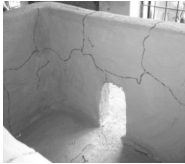
Figure 15: Position of crack formation in reinforced experiment.
