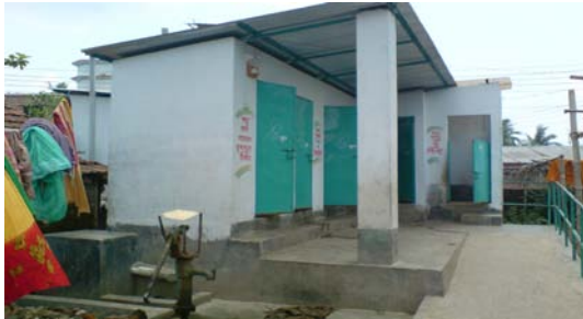
Figure 1: Constructed community latrine in Montu colony slum (2009), where community contribution was Tk. 14,616 and the ASEH grant was Tk. 1,62,168.
