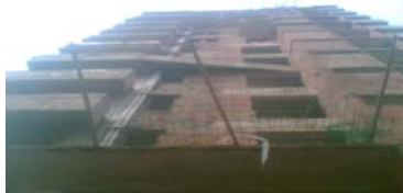
Figure 1: This is a figure of using inadequate safety net in a high-rise building at Zindabazar site
