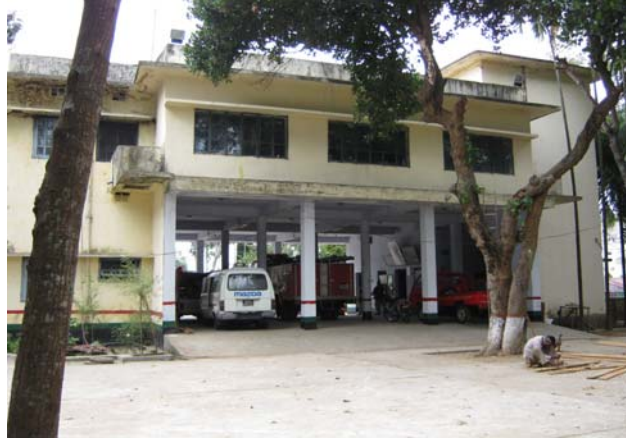
Fig 4: Soft storey found in surveyed building in Rangamati.
