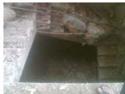
Fig-3: Cavity in the stair room, there is no safety fence around it, so accident can take place any time.
