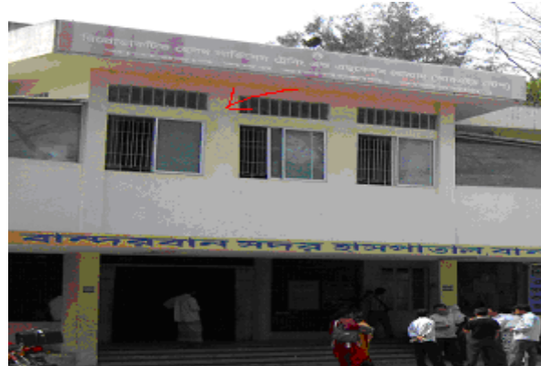
Fig 6: Short column found in the surveyed building in Bandarban.
