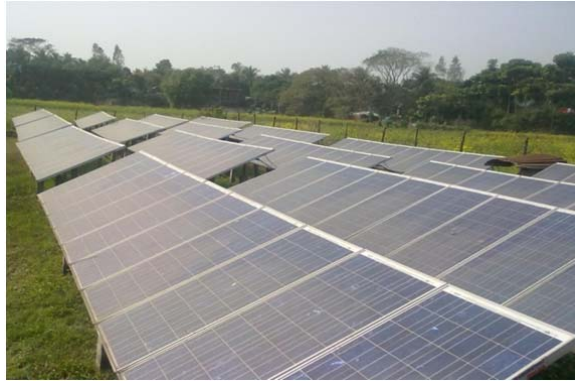
Fig 4: Solar water pumping demonstration project in Savar, Dhaka
