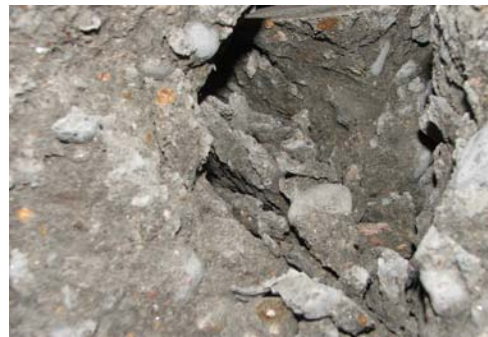
Fig-5 (c): Polymer cement concrete after failure
