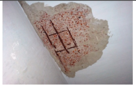
Fig 2: Leakage of slab cause rainfall intrusion
