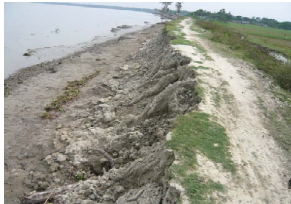
Fig. 5 (a) Typical embankment section (h = horizontal; v= vertical; T= top width; w= base width; H= height of the embankment; β= slope angle) and (b) eroded embankment section due to wave action.
