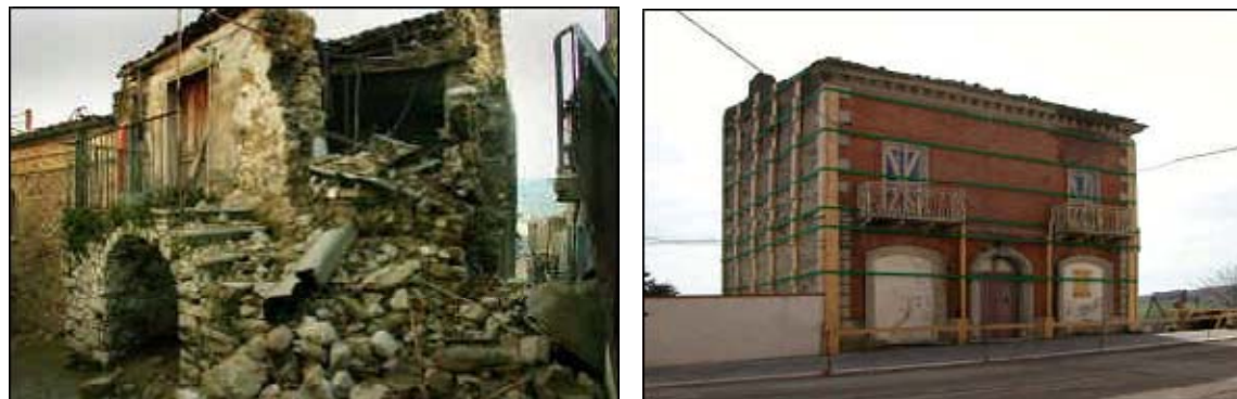
Fig. 5: (a) Collapsed Walls in historic citadel, (b) Little damaged building with Nylon straps (Italy 2003)
