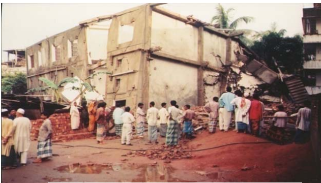
Fig.3. Building failure in Kalabagan
