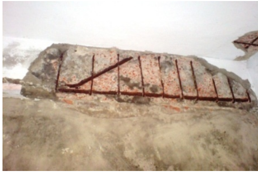
Fig 1: Falling down of plaster from a beam section
