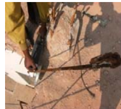
Fig 5c: Curtailment of corroded reinforcing bar
