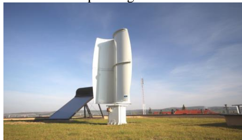
Fig. 8: Wind turbine with vertical axis
