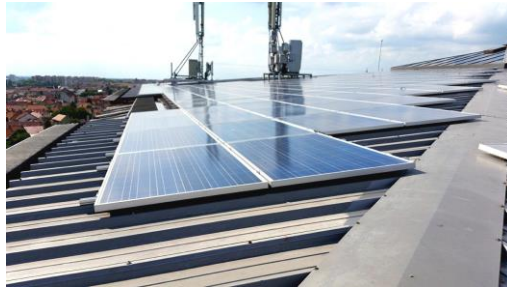
Fig. 4: Photovoltaic on grid system 161 kWp.
