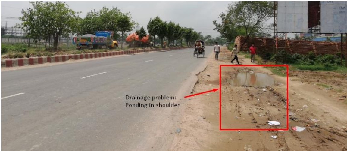
Fig. 1: Drainage Problem and Damaged shoulder near Amin Bazar Bridge (Dhaka-Aricha Highway)
