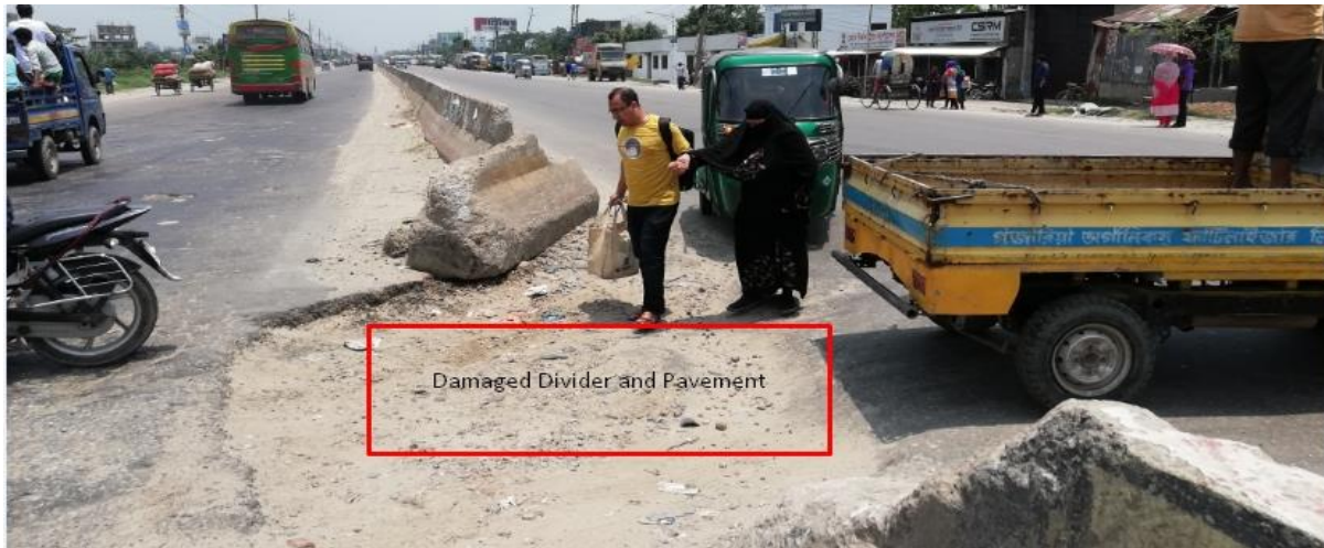
Fig. 4: Damaged Road Divider- through this vehicle moving and damaging pavement and pedestrian crossing road risking life in front of Samsul Hoque Khan School and College (Dhaka-Chittagong Highway)
