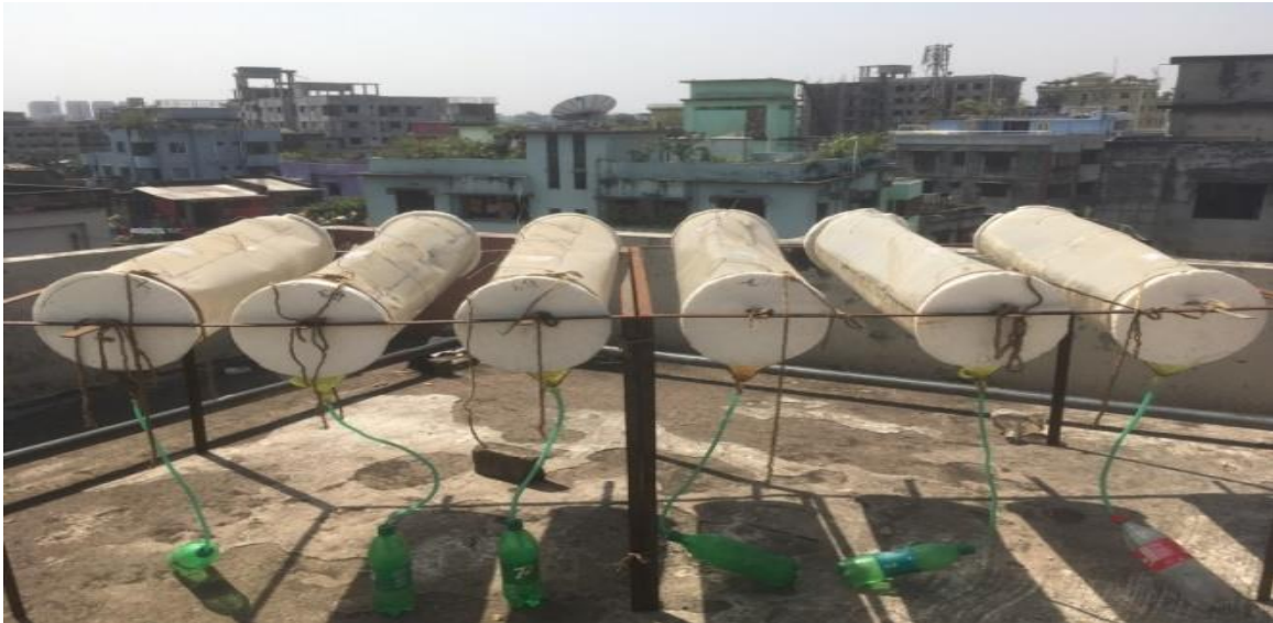
Figure 5: Placement of final model at roof top.
