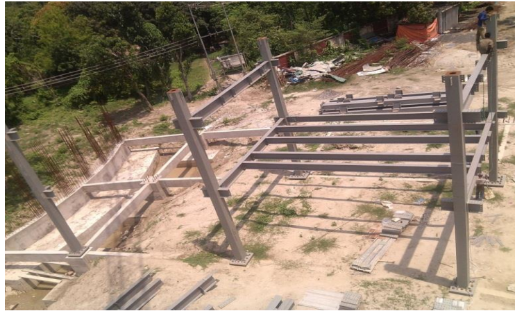
Figure4: Concrete-Filled Fabricated Steel Box Composite Column (FSBCC) Bachelor Quarter, Air Force Base, Joshore Bangladesh 2017
