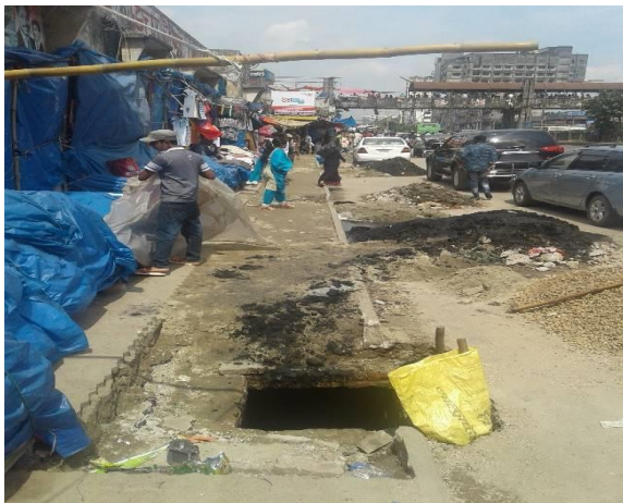
Figure 7: Open drains on footpath in Dhaka city
