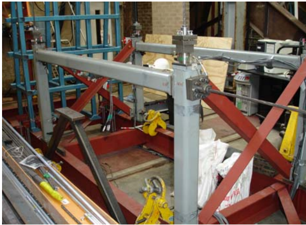
Figure 9: Self centering frame being prepared ready for installation of damper element at the top of inverted 'V' bracing.
