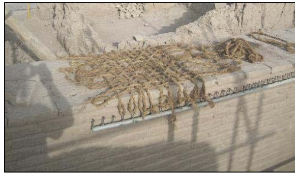
Figure 7 Horizontal Siess, simulation process with available thick elements in site just for learning the implementation adjustment (the main useable Siess will be strongly thinner)
