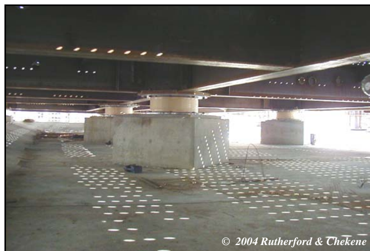
Figure 4. Photograph of a typical rubber bearing on a concrete pedestal in the crawl space, new de Young Museum.
