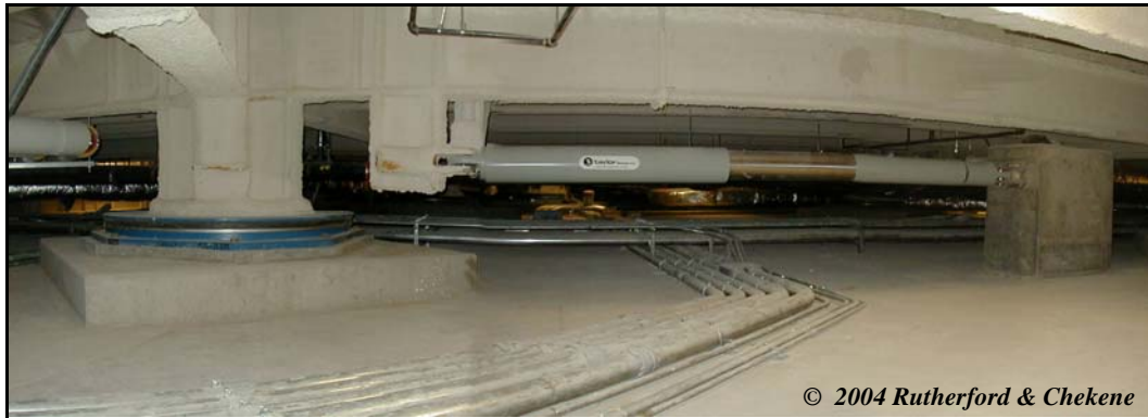
Figure 5. Photograph of a typical sliding bearing and fluid viscous damper in the crawl space, new de Young Museum.
