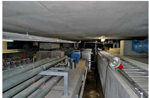
Base Isolation Floor
