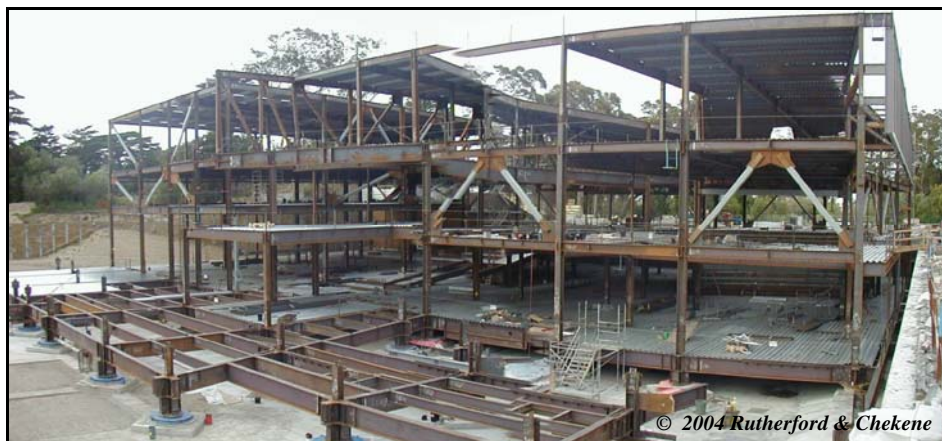
Figure 3. Photograph of the new de Young Museum during construction, showing foundation, isolation system and steel framing erection.
