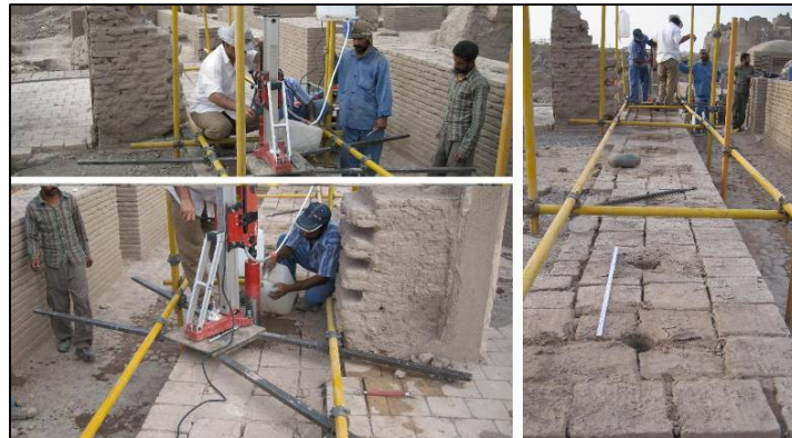
Figure 6 Drilling procedures for inserting vertical Siess elements in main walls of Pyambar Mosque
