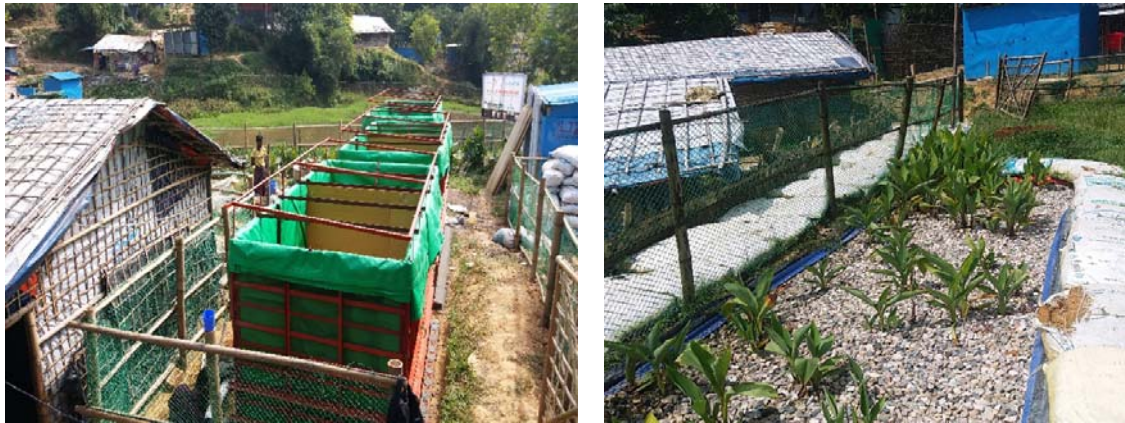
(a) (b) Figure 9 (a) Filtration chamber (b) Constructed wetland of PA FSMU
