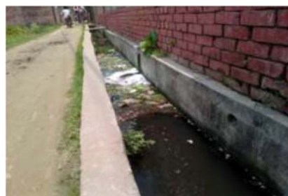
Figure 5 Blocking of drainage
