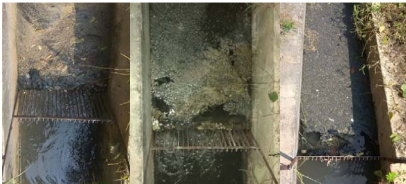
Figure 5 Observation of the drain after 1, 12 and 24 hours of installing the bar screen.
