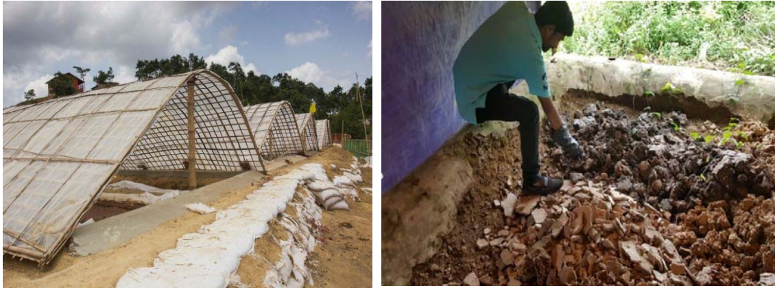
Figure 11 (a) Sludge drying bed (b) Dried sludge stored in the house of UKAID FSTS
