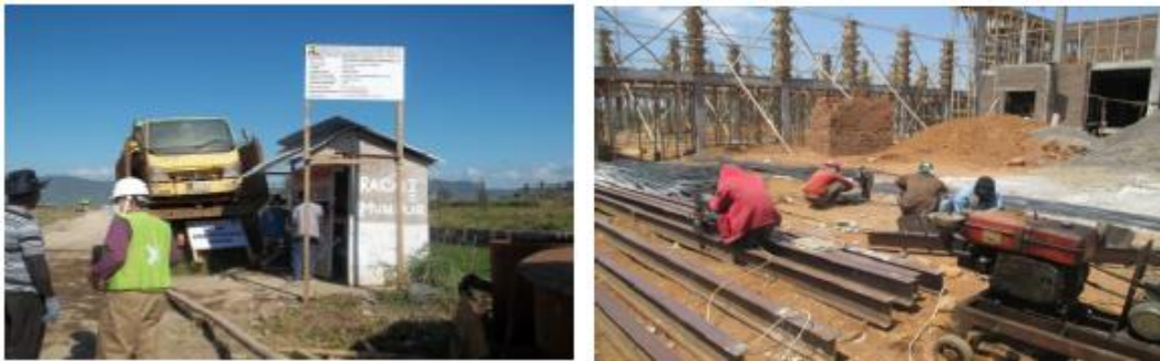
Fig 6 and 7 unsafe condition in construction project
