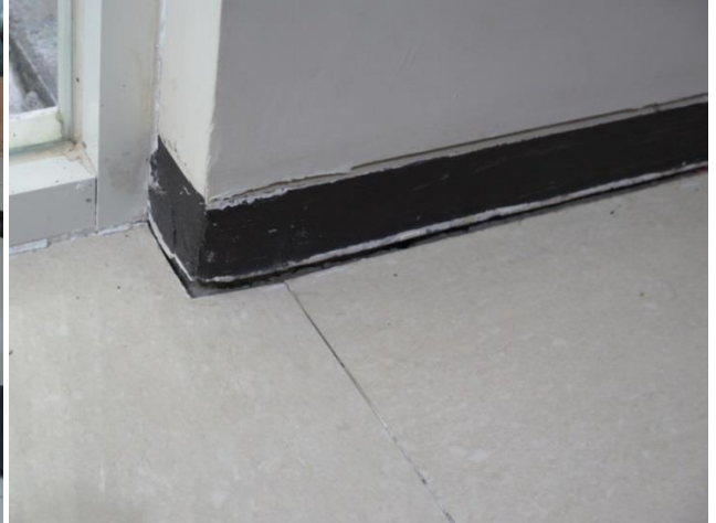
Fig. 6 Gap between floor and wall
