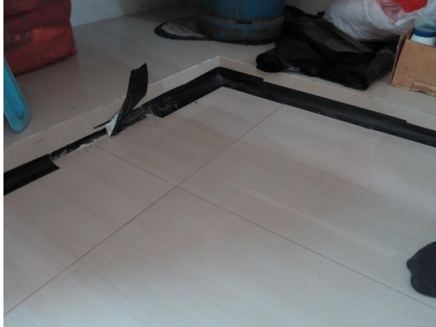
Fig. 5 Differential settlement of floor
