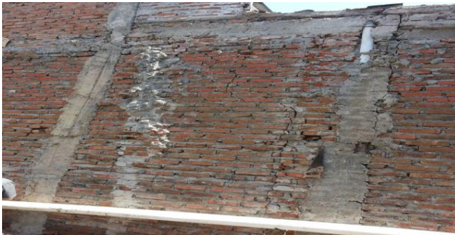
Fig. 11 Poor detailing at beam-column joint
