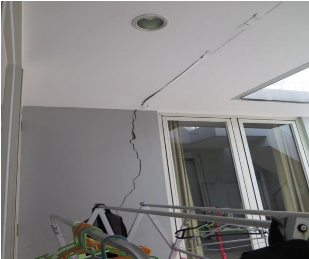
Fig. 9 Diagonal crack on the wall and ceiling
