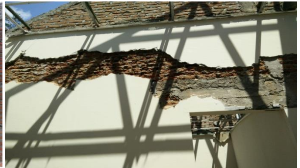
Fig. 12 Poor detailing of beam-column joint and horizontal cracks on the brick wall
