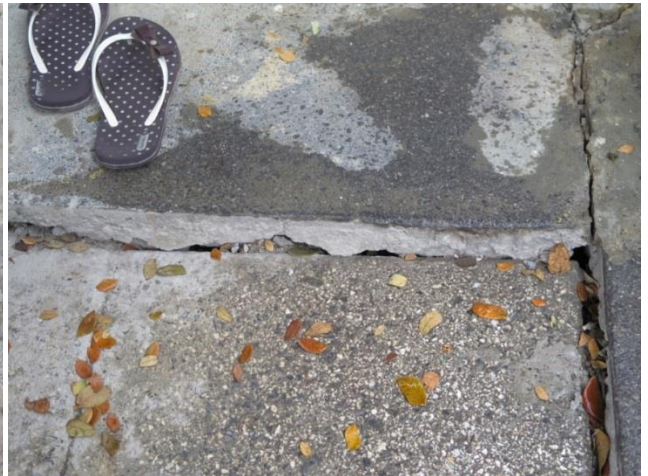
Fig. 8 Crack and differential settlement of unreinforced carport slab
