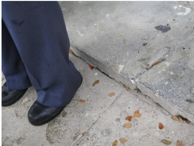
Fig. 7 Differential settlement of carport slab
