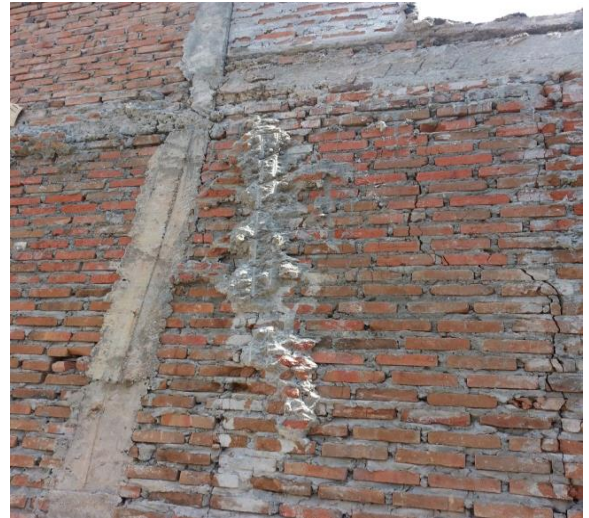
Fig. 10 Vertical cracks on the brick wall
