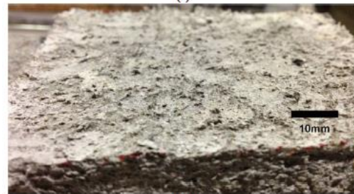
Fig. 11. PCM surface deterioration (flakes dropping) after FTC: (a) External surface, (b) Interface
