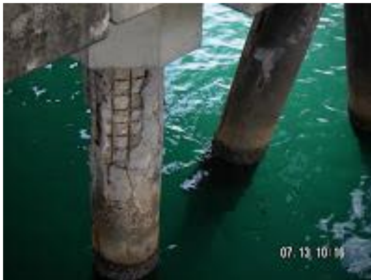
Fig. 1. Corroded rebar in piling.
