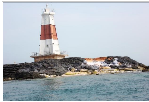
Fig. 2. Damage Point Batu Berhanti Island Coastal Protection.
