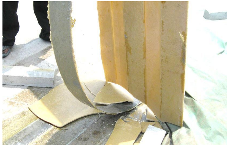
Figure 9: Debonded CFRP and mortar grout after a few days of 1 st trial repair.
