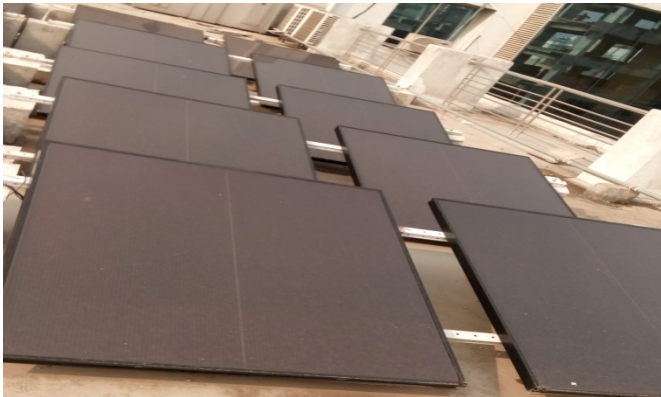
Fig. 2 Thin Film solar PV array
