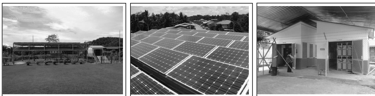
Fig. 3. (left) Solar PV structure and power house at SK Labuk Subur, (centre) solar PV panels at SK Sungai sungai, (right) system power house for batteries, inverters, diesel generator and other accessories at SK Lung Manis.
