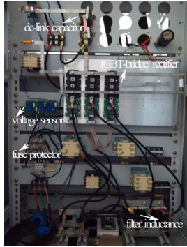
Fig. 9. The experimental platform of the PWM rectifier.
