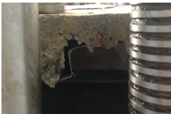
Fig.12: Concrete cover separation
