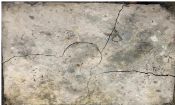
Fig.10: Failure modes of slab under loading
