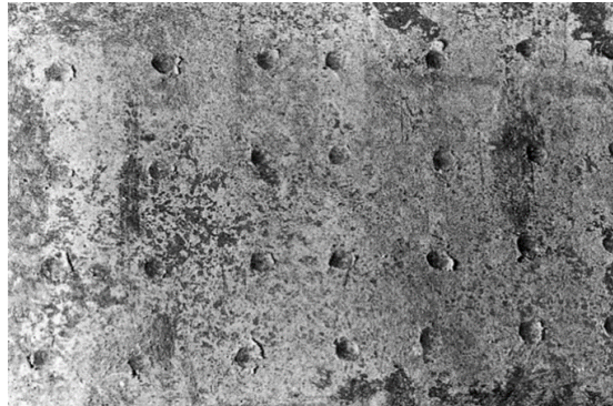
Figure 2.27: Surface damage on green concrete (Bungey and Mandandoust, 1994)
