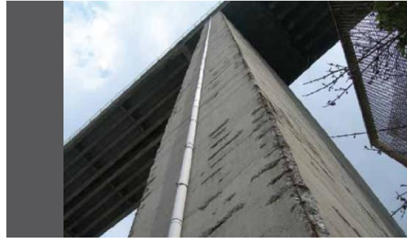
Figure 2.1: Carbon deteriorated concrete (MAPEI SpA Manual, 2021)
