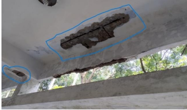
Figure 4.4: Spalling and leaching shown in beam and floor slab concrete with corrosion of rebar
