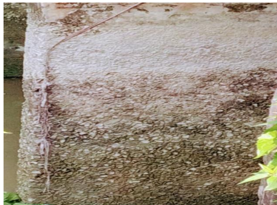
Figure 2.3: Typical state of deterioration of concrete by chloride attack (Part of bridge structure at seawater contact)
