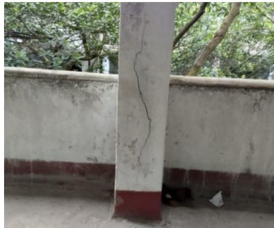
Figure 4.3: Cracks seen in column concrete of the structure
