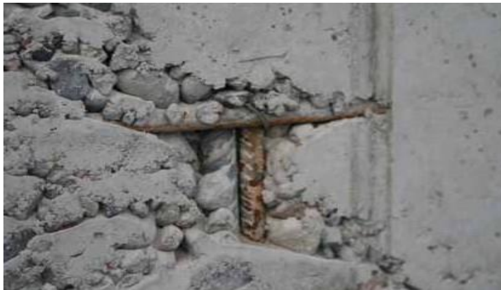
Figure2.10: Segregation of aggregates, a symptom of incorrect casting of the concrete (MAPEI SpA Manual, 2021)
