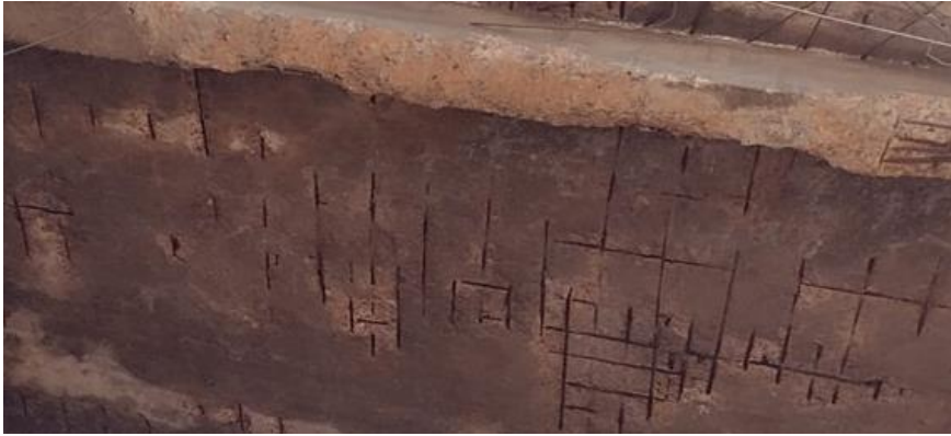
Figure 2.19: Steel industry premises concrete spall by carbon attack.
