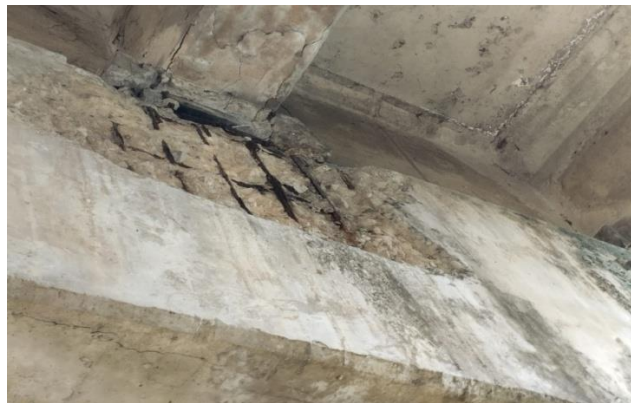
Figure 2.5: RCC bridge girder concrete spalling due to load impact at support zone.
