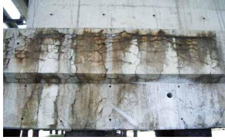
Figure 2.4 Deterioration due to alkali-aggregates reaction (MAPEI SpA Manual, 2021)
