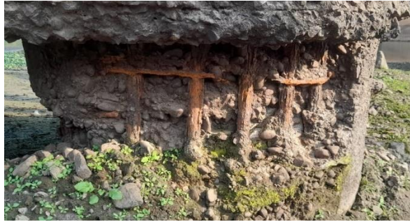
Figure 2.7: Erosion due to high speed of water flow of RCC situ-pile concrete
