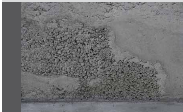
Figure 2.8: Segregation of aggregates due to incorrect preparation or casting operations (MAPEI SpA Manual, 2021)
