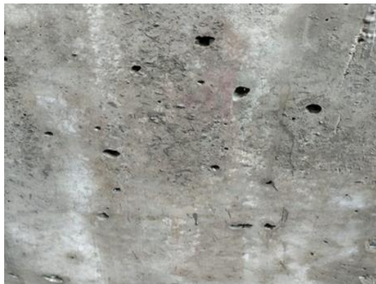
Figure 2.9: Concrete honeycomb in a newly constructed structure
