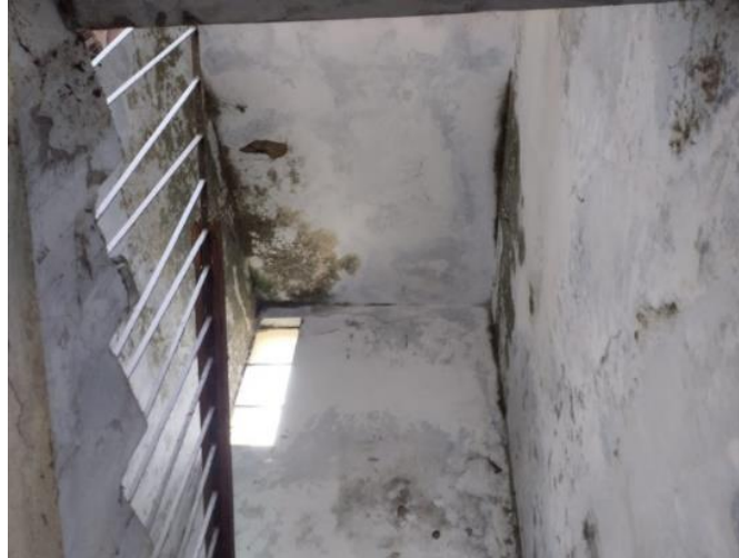
Figure 4.6: Weather damp shown in slab, wall, and beam concrete of the structure
