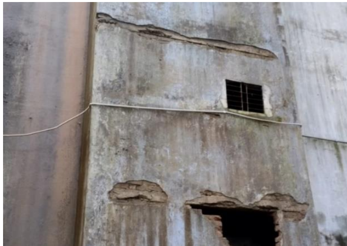
Figure 4.5: Distresses shown in beam and floor slab concrete outside of the structure
