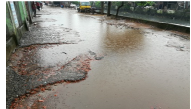
Fig. 9: Road damaged by water logging
