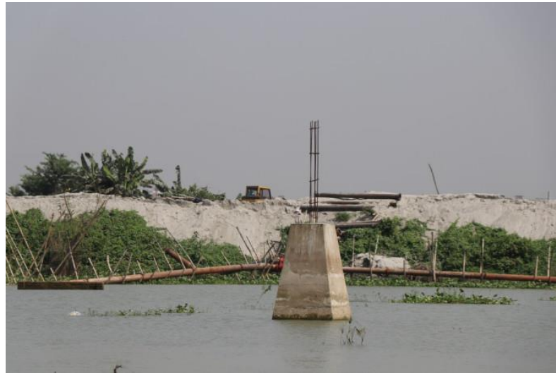
Fig 4.9: A submerged RCC demarcation pillar of Turag river boundary
