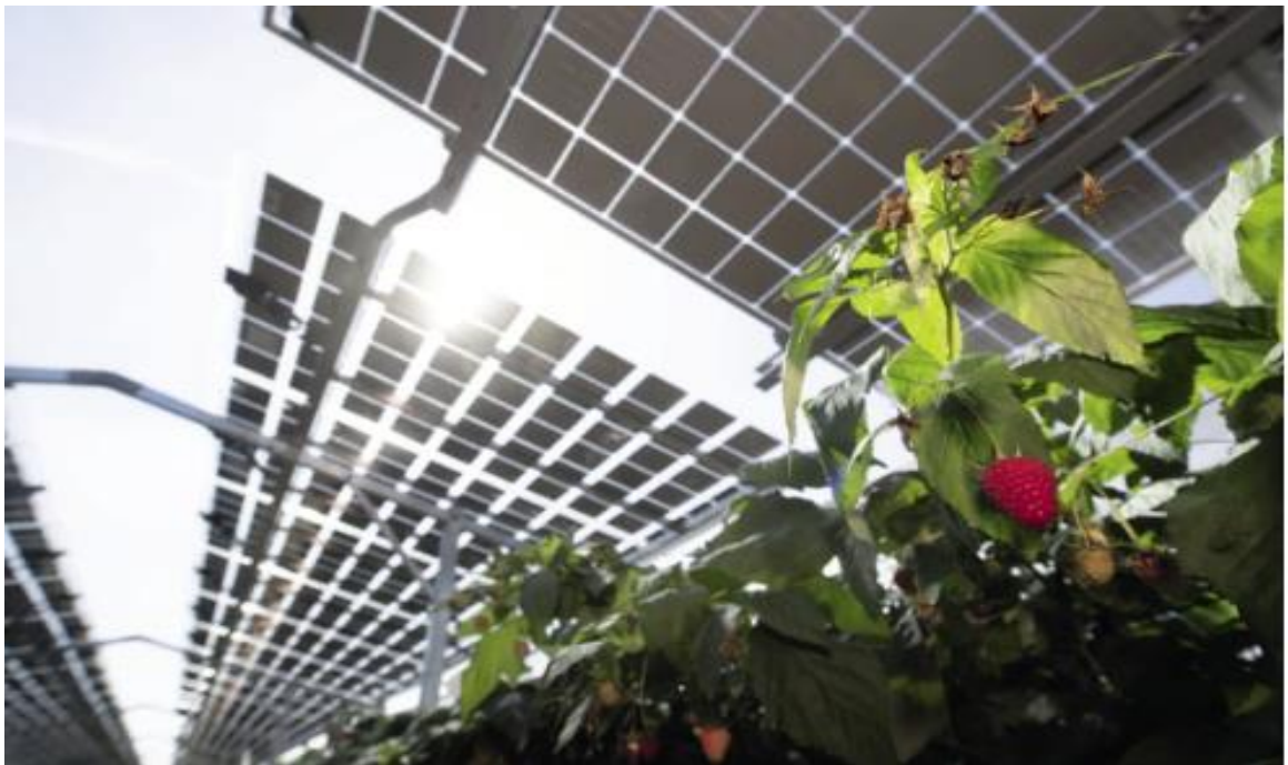
Fig. 2.11: Sits of 3.77 MW Soudia Agro Solar PV Power Plant [84].
