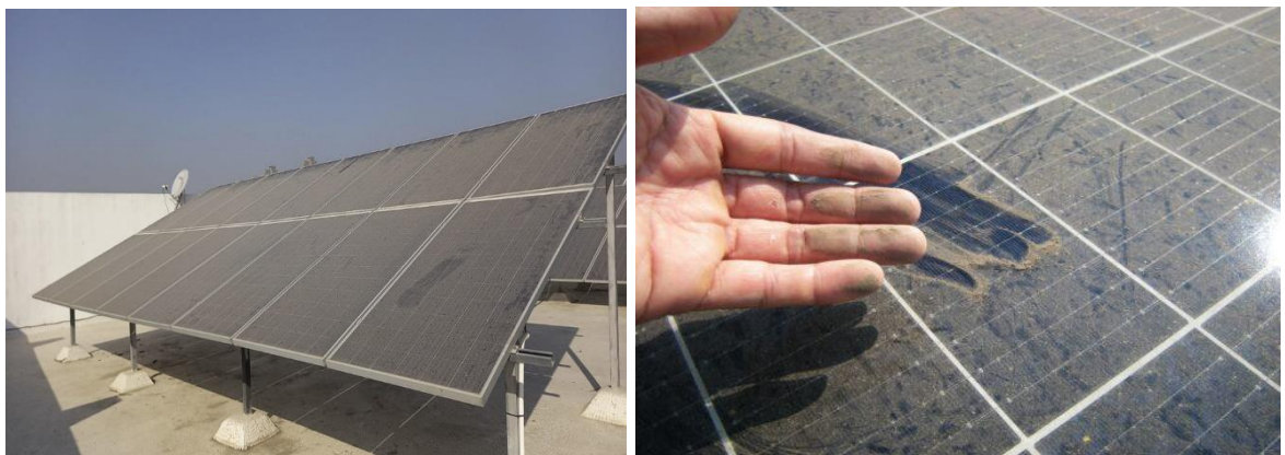
Fig. 5.15: Dust accumulation on solar panel
