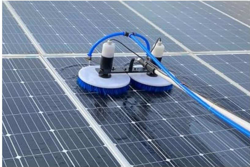
Fig 4.7. Solar PV cleaning using automated brushes
