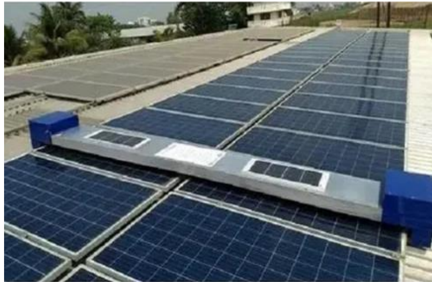
Fig. 4.4: Battery-operated automatic wiper-based cleaning.
