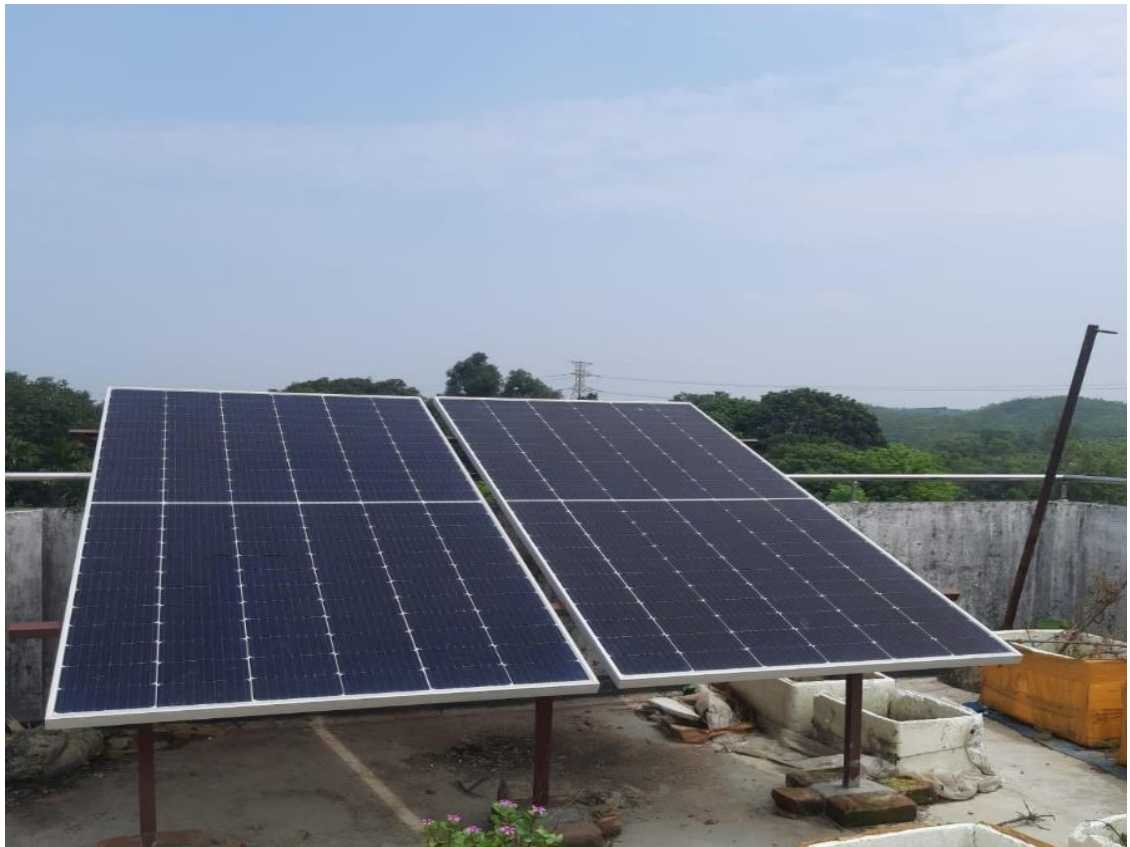
Fig. 3.4: Set up of solar PV system
