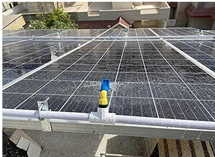
Fig. 4.5: Automatic solar panel water cleaning system.
