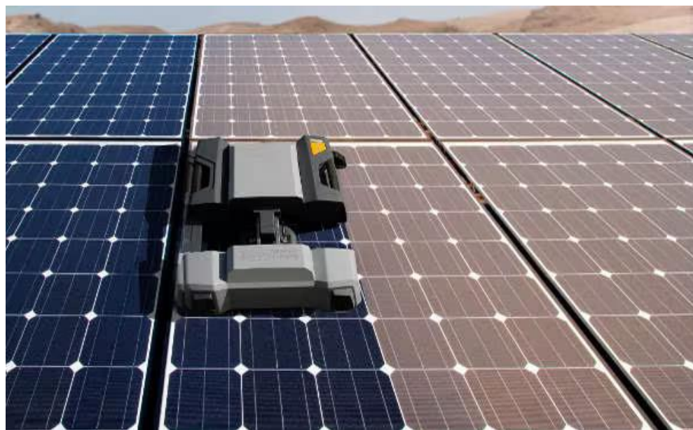
Fig. 4.6: Automatic solar panel water cleaning system.
